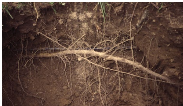
Figure 6. Root concentration around a subsurface drip line. (Photo by L. Schwank)
