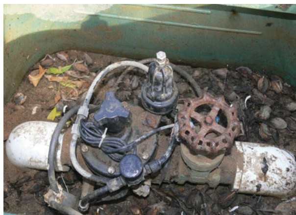
Figure 14. In-field pressure regulator used to regulate the pressure to a block of the orchard. (Photo by B. Sanden)
