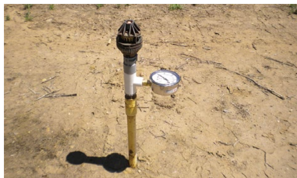
Figure 10. Rotator sprinkler with pressure gauge attachment temporarily installed during field evaluation to measure the pressure at the sprinkler head.
