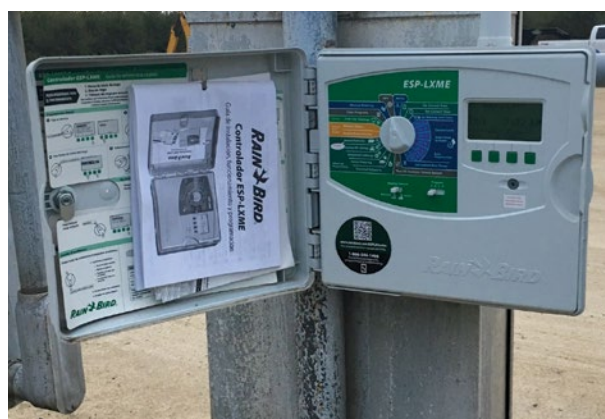
Figure 3. Controller for an automated irrigation system. (Photo by S. Cooper)
