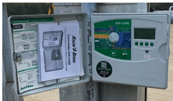
Figure 3. Controller for an automated irrigation system. (Photo by S. Cooper)
