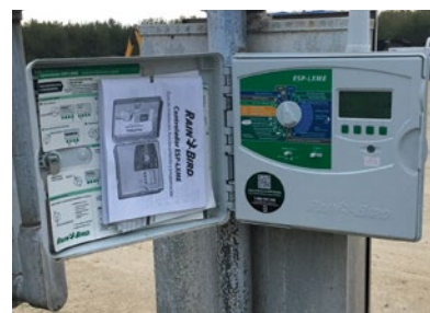
Figure 1. RainBird LXME Pump and Valve Controller. (Photo by S. Cooper)
